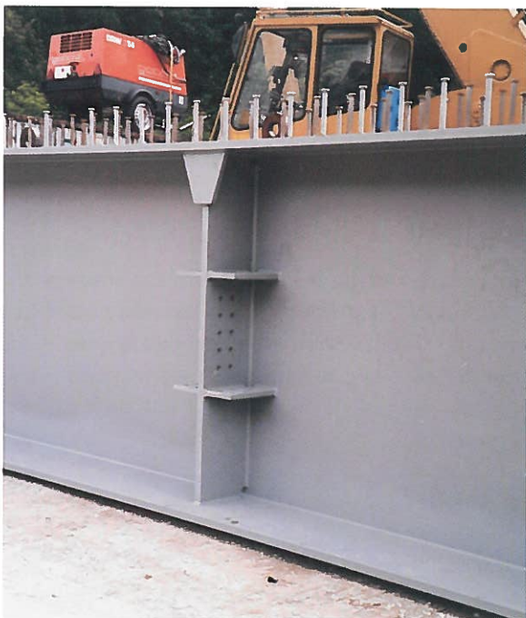
Photos 17a : Montant courant / Current vertical stiffener
